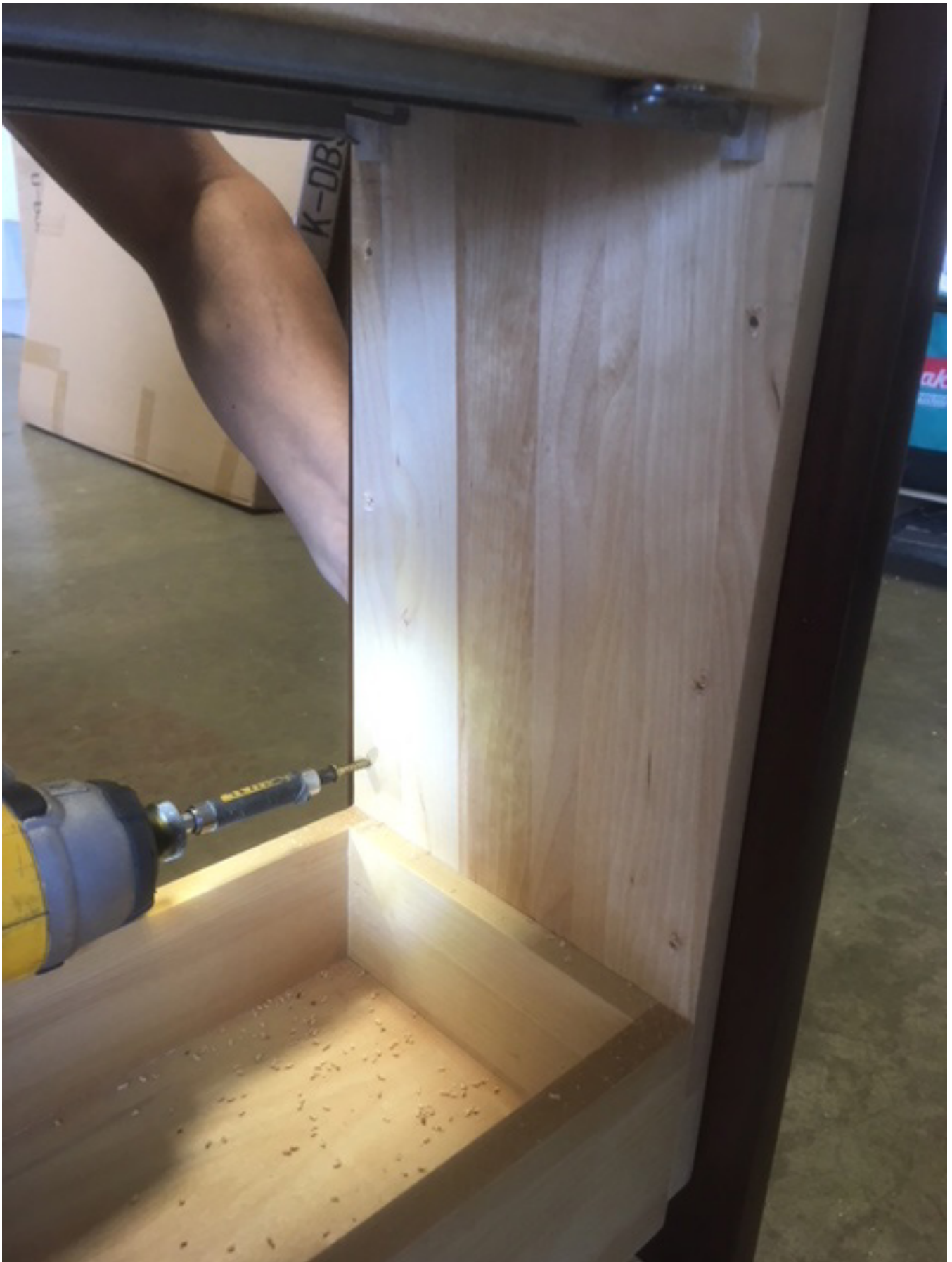
Six holes for the bottom part, two holes for the top part.
